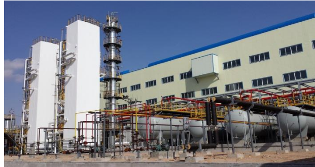
1 million Nm 3 /day LNG Plant in Alashan
