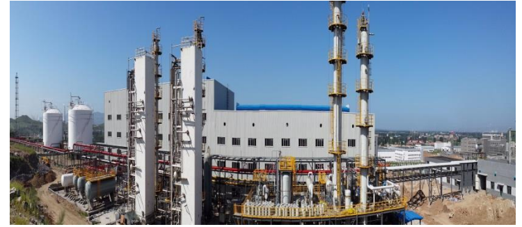
1 million Nm 3 /day LNG Plant in Zhangjiakou
